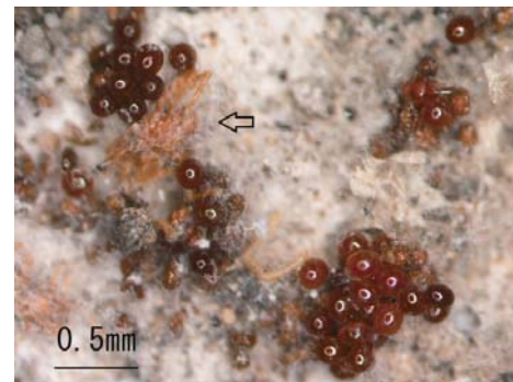
Fig. 4 Mite eggs laid on a thin concrete piece attached to an about 40-year-old concrete wall (G26-1). An arrow shows a dead adult mite near eggs.
