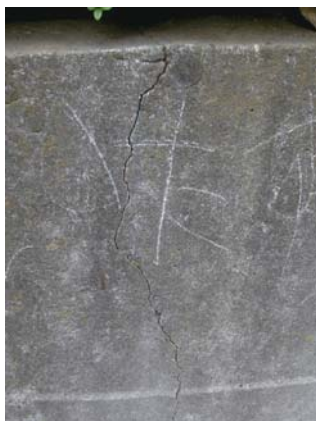
Fig. 3 Crack of an about 15-year-old concrete wall on the ground (G20). Many mite eggs were collected from it.
